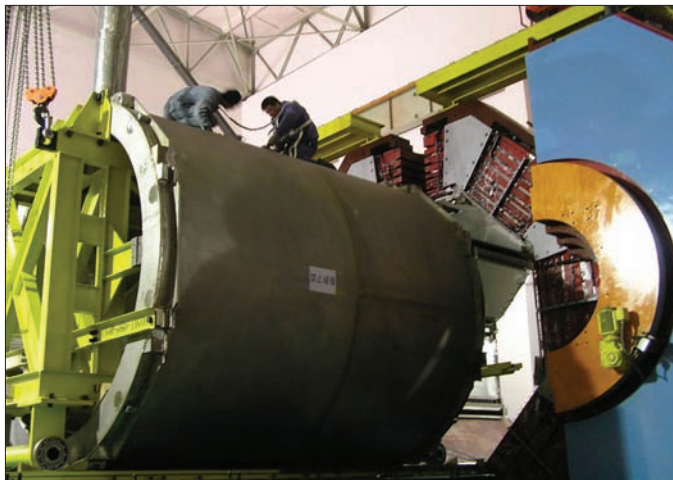
Fig. 5. The superconducting magnet coil during installation into the BES III detector. The next stage is to cool the magnet.
